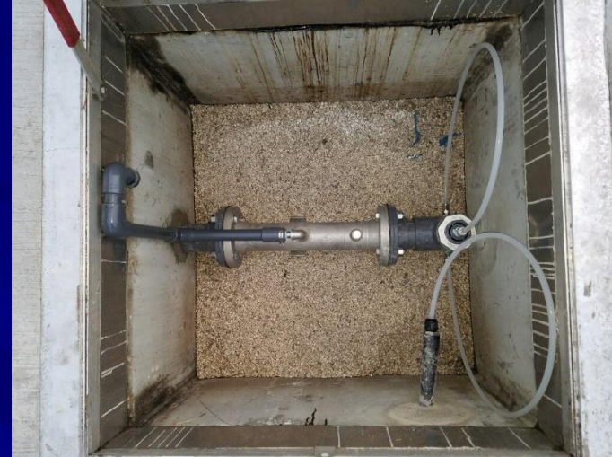
Venturi for Air Addition
